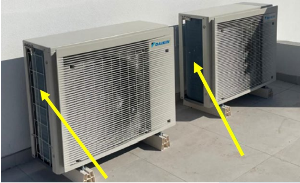
Outdoor units, with and without the inlet grilles
